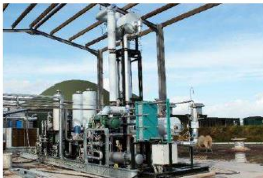
CO 2 Liquefaction Unit
