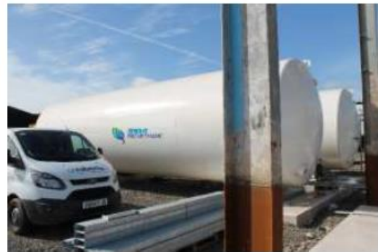
Horizontal CO 2 Storage
