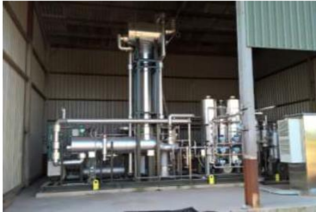
CO 2 Liquefaction Unit
